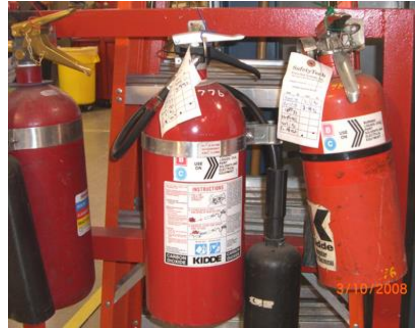
Fire Extinguishers (20# Size shown)
